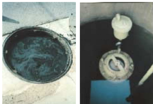
Figure 2. Submerged air release valve
